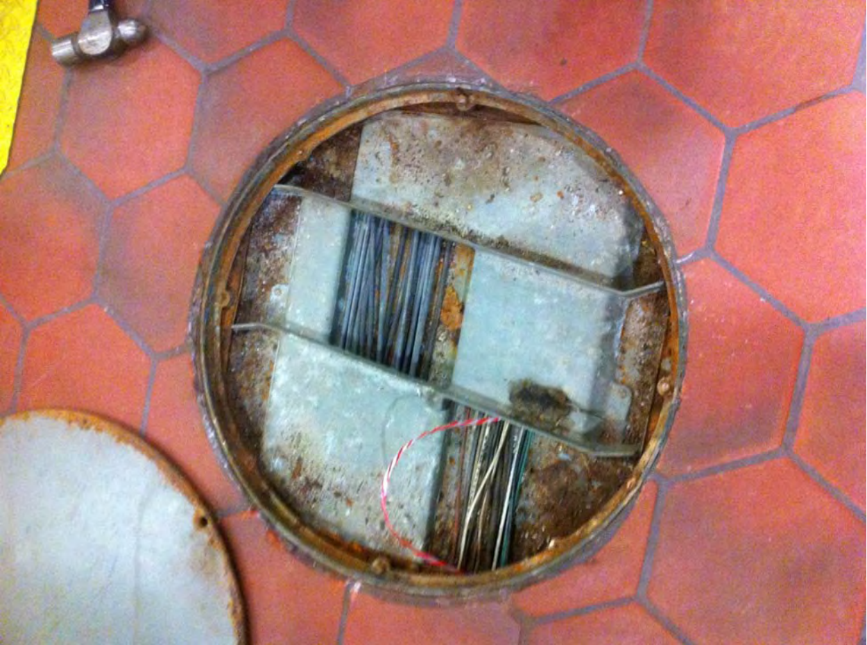
Photo #2 - Hand Hole 1 in good condition and not at capacity
