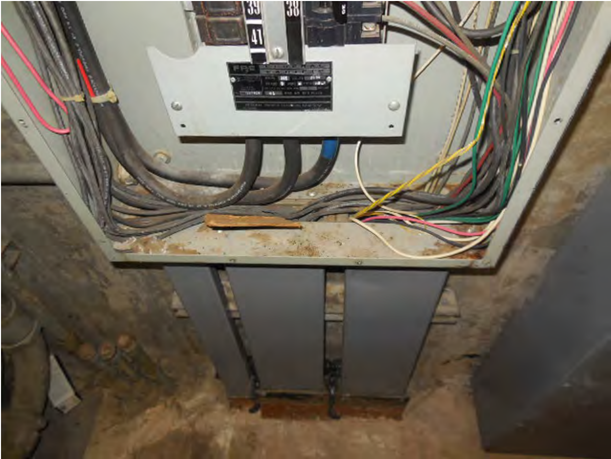
Photo #4 - Walker duct connection to AFC Panel in Room C108
