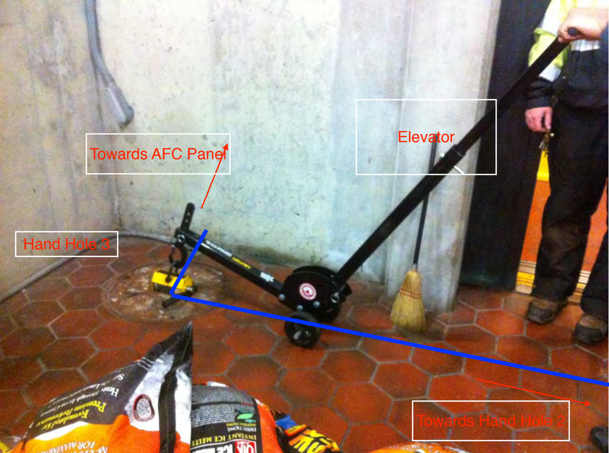
Photo # 3 – Hand Hole 3 under Salt Box and adjacent to elevator.
